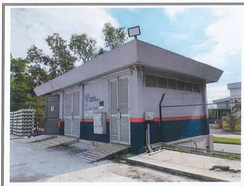
VIEW OF THE TNB SUB-STATION
